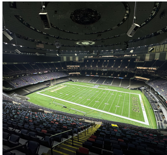
Verizon 5G antennas inside the stadium. Image credit: Verizon
